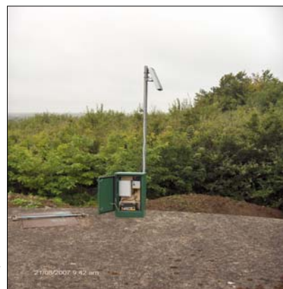
Solar power installation in Ireland
